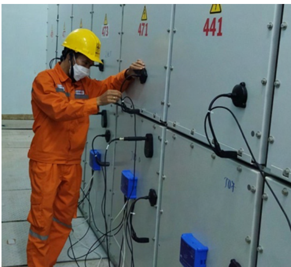
Dak Lak High Voltage Grid Operation Management Team inspects discharge at 110kV Ea H'leo substation
