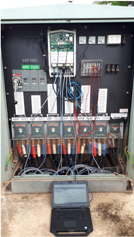
VisNet being commissioned in a kiosk substation
