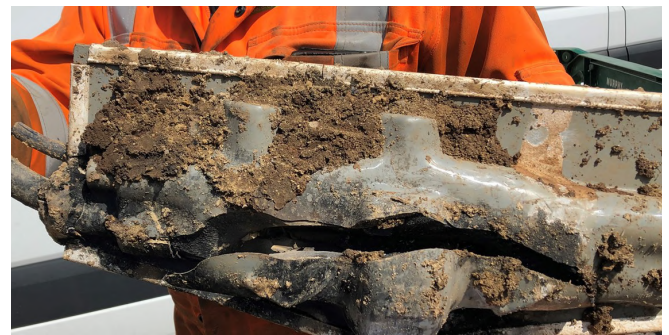
Faulty LV joint taken from service prior to failure
