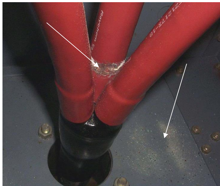
Figure 1 Surface discharge activity between cable phases.
