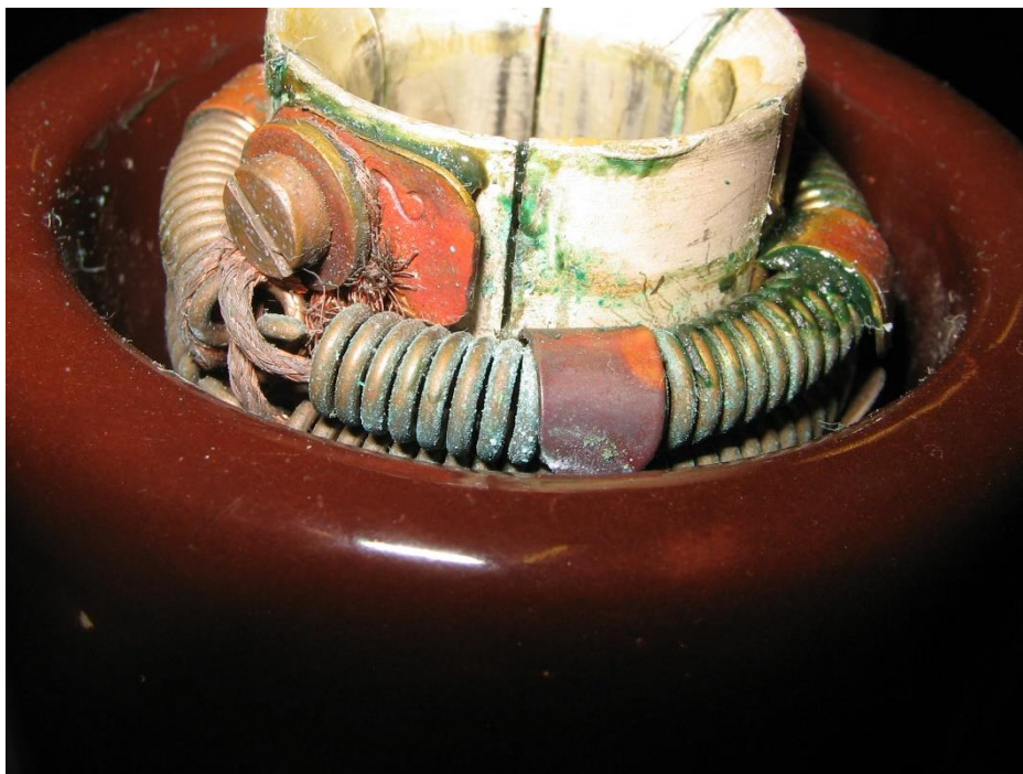
Figure 7 Evidence of discharge activity within a porcelain contact cluster of an 11kV circuit breaker.
