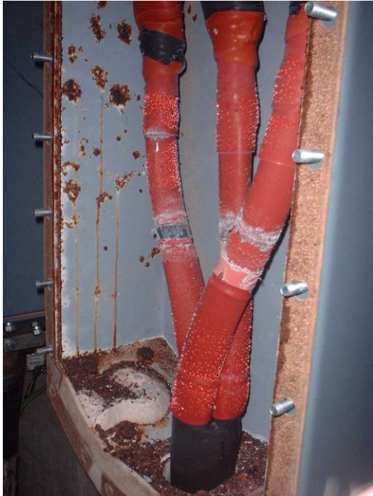
Figure 2 Evidence of advanced discharge activity within an 11kV switchgear air insulated cable box.
