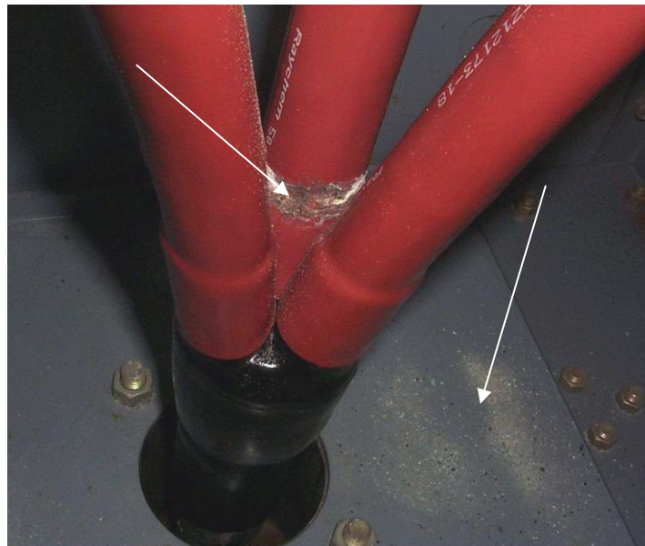
Figure 1 Surface discharge activity between cable phases.
