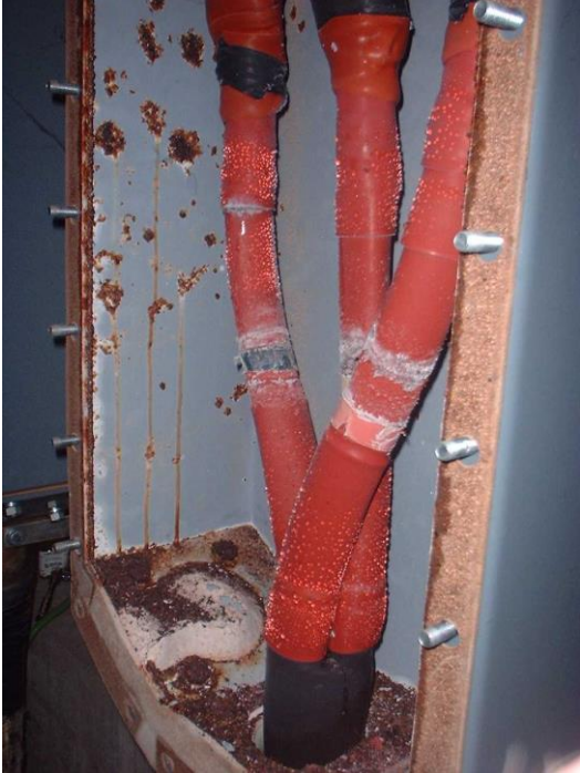
Figure 2 Evidence of advanced discharge activity within an 11kV switchgear air insulated cable box.
