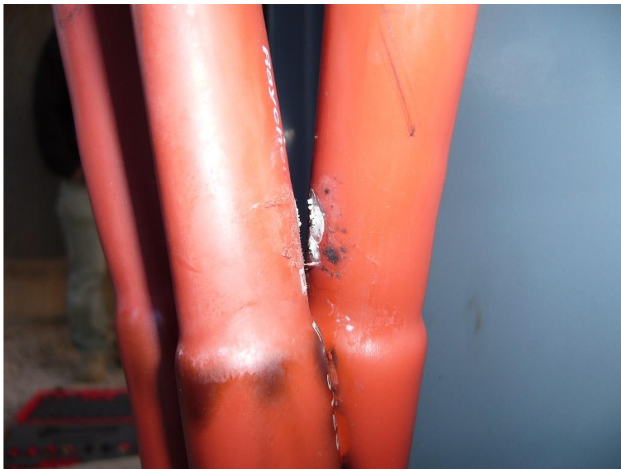
Figure 3 Discharge activity between cable phases within an air insulated cable box. Note white powder deposit on polymeric surfaces.
