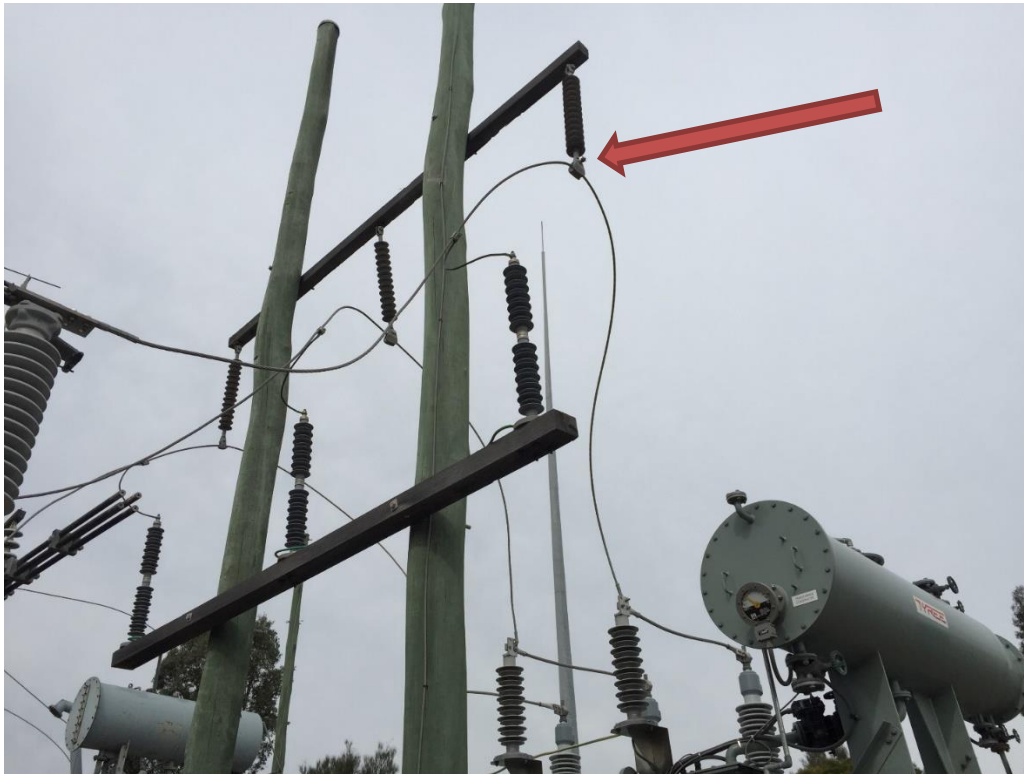
Figure 7 North phase 66kV dropper at TX021
