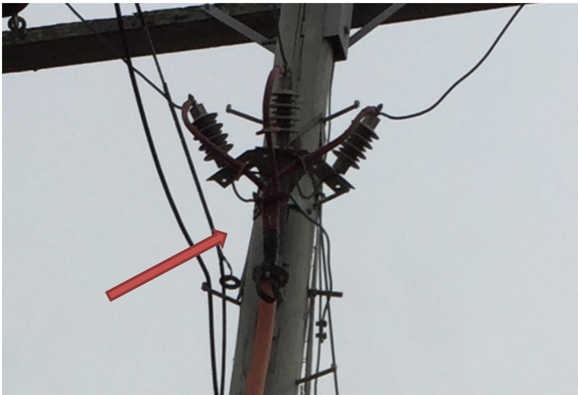
Figure 17 Cable head termination 54100
