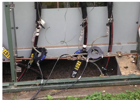
Figure 4: RFCT Sensors Installed on Ground Straps
