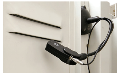
Figure 2: Ultrasonic Sensor Mounted Outside Cubicle
