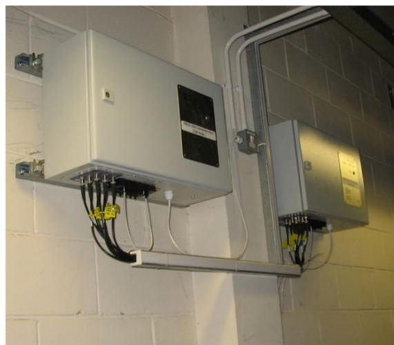
Figure 4 CDM Measurement Nodes Mounted Within Substation
