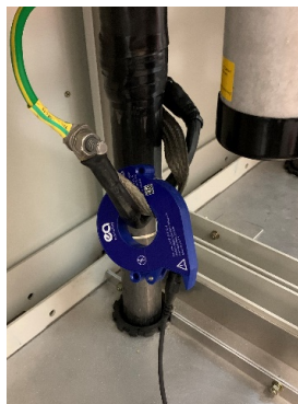
Figure 1 HFCT around earth sheath
