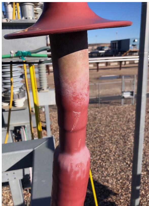
Cable termination H3 with uneven contamination
