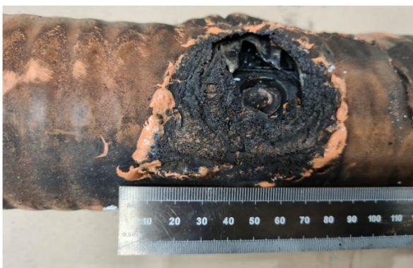
Figure 1: Failed cable section as received
